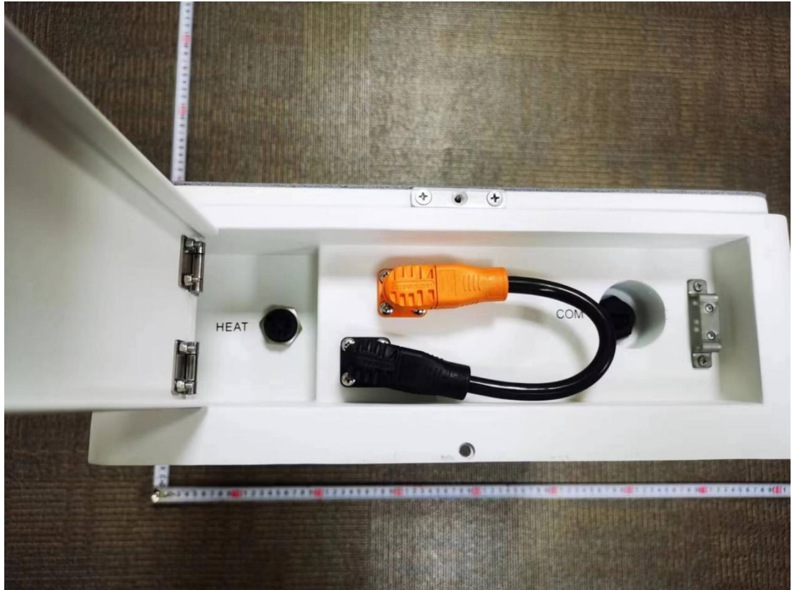
Communication connection of Main control unit
